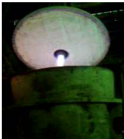
Fig. 4. View of the mixed recuperative installation (recuperative burner with recovery device mounted in the ladle lid)
